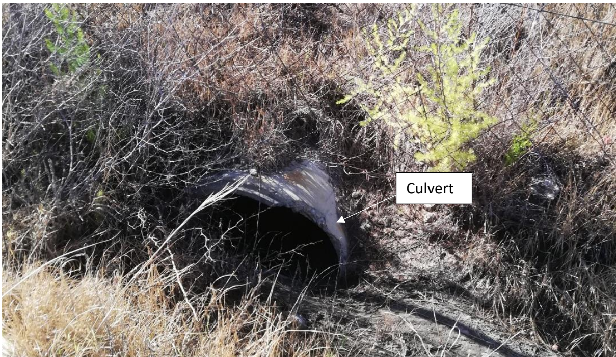
Plate 2-3 Example of a blocked culvert along the original drainage line
